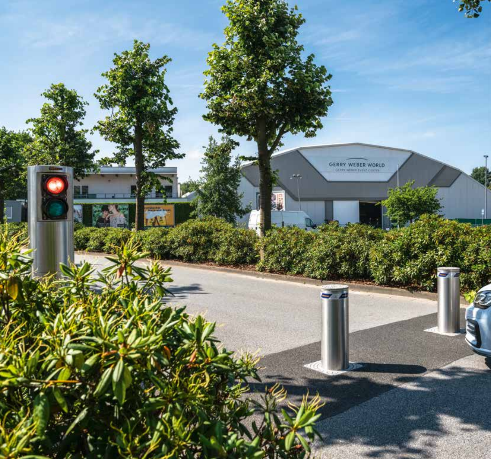
TOP LEFT. Automatic bollard with hydraulic operator
